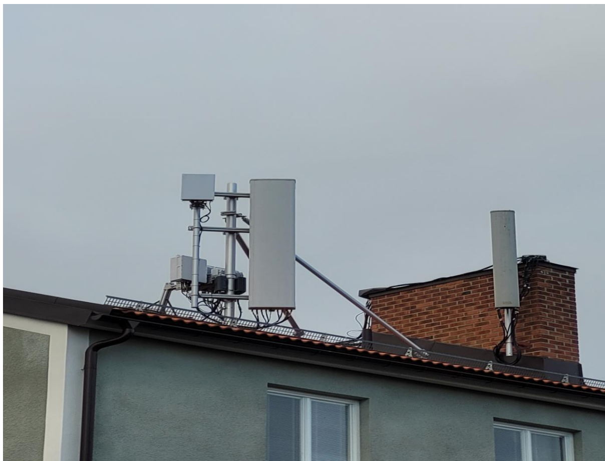
5G base station on the roof of a three floor building located 60 meters from the study apartment. Initial figure after the 5G installation showing the previous base station attached to the chimney
