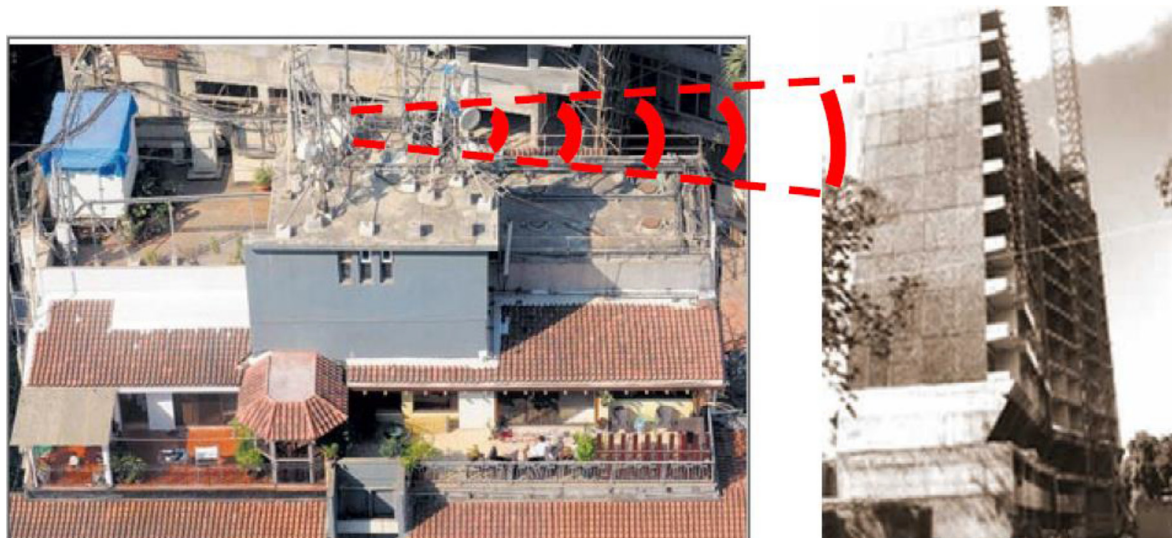
Fig. 3. Mobile towers installed on Vijay Apartments terrace at Carmichael Road, Mumbai.
