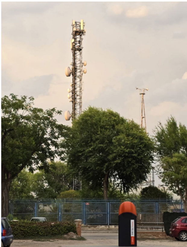
Fig. 7 Telecommunications antenna in the blue zone of Figs. 5, 6, 8, 9, and 10. The mast supports the antennas of different mobile telephone operators. In the foreground, the exposimeter is shown in the measurement process
